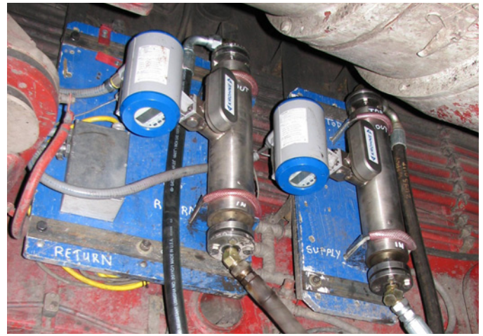
Figure 2. Truck-Mounted Krohne Coriolis Mass Flow Meters
